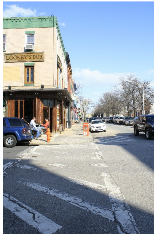
Faded crosswalk in Canton
